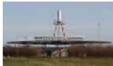
Fig: 12.28 A VOR system installed at airport maintain a highly reliable, safe, and efficient ground-based navigation system.
