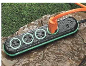
Fig: 15.24 Electrical extension placed damped environment
