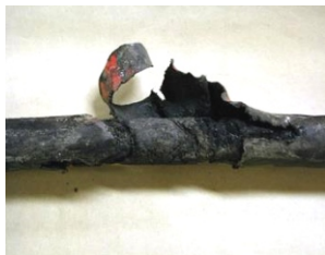
Fig: 15.23 Over heating of a cable
