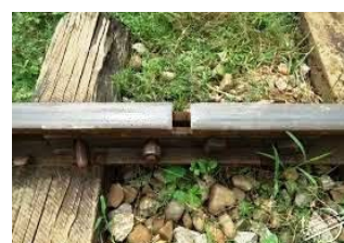
Fig (9.13) Gaps between Rail Tracks
